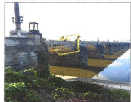
Picture shown is TEN installing LED bridge under-lighting for the City of Harrisburg in November, 2016. The LEDs have controls and will be programmed for 26 different color sequences for special occasions such as Red, White and Blue for the 4 th of July. This is the “icing-on-the-cake” as 6,000+ streetlights already have been installed across the City.
