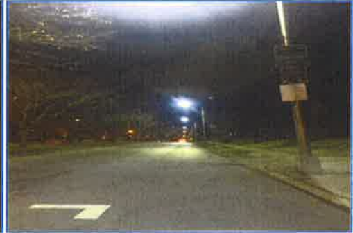
Baltimore After – LED Cobra Head Luminaires
